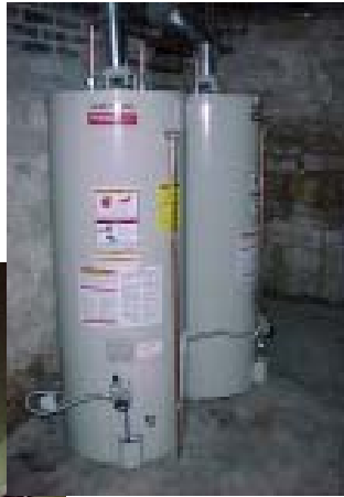
Above: Two new hot water heaters replaced the aging one, providing the necessary amount of hot water to serve the upgraded bathroom facilities.
